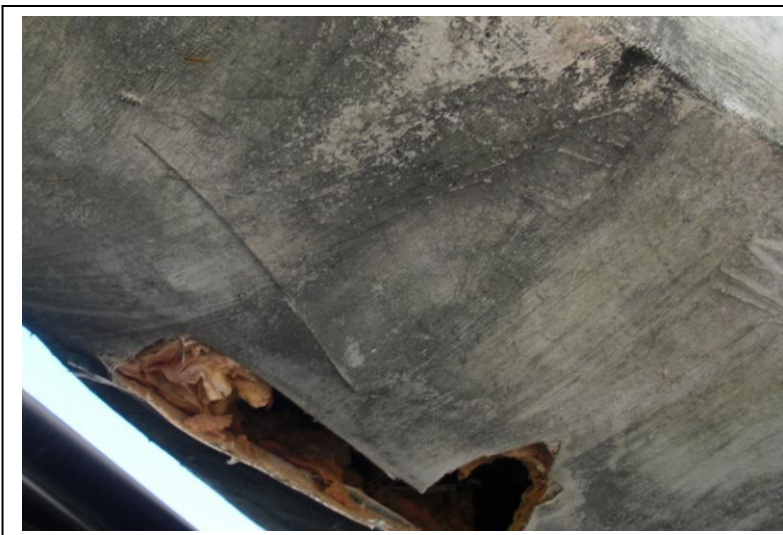
Moisture has broken through seal layer
