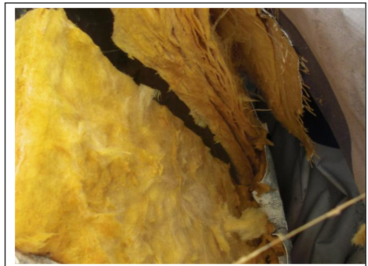
Wet insulation at unit discharge
